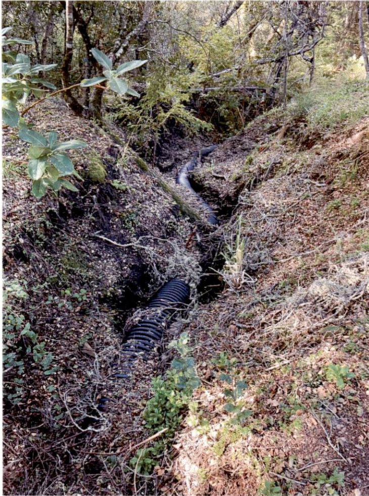
Photo 6 — Looking southwest, a Culver contains a black pipe that flows into La Honda Creek that occurs downslope from the scene at 10707 La Honda Road, Woodside, CA 94062 (San Mateo County) (Assessor's Parcel 078-190-210). As mentioned in the text above, the Culver's bed and top of banks do not host wetland/riparian plant species.
