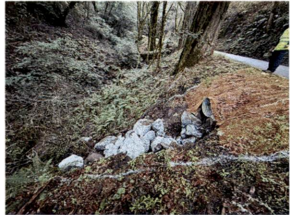
Photo 1. Slip-out facing east (2/20/2025).
