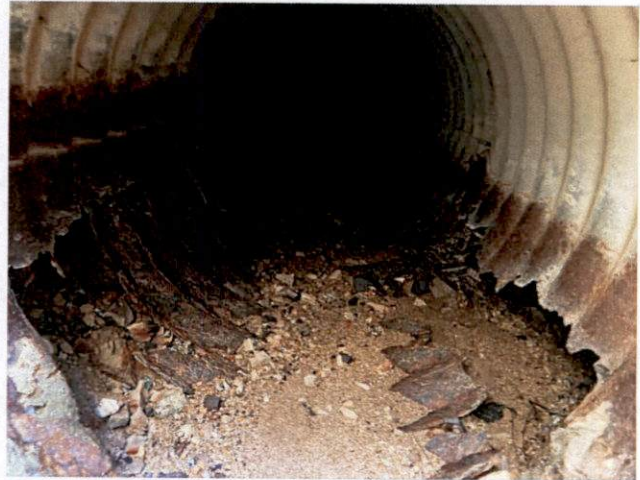
Photo 1. Mile 4.7 deteriorated culvert (February 18, 2025).
